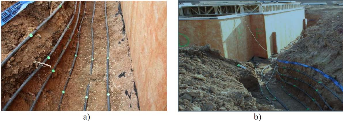
Figure 2 FHX in a) basement excavation, b) extended into utility trench (Courtesy: Piljae Im, ORNL)
