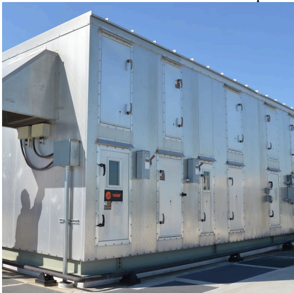
The dedicated outdoor air system.
