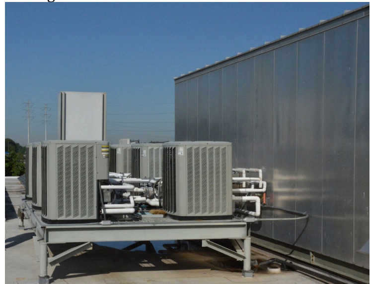
The condensing units for the DOAS system.
