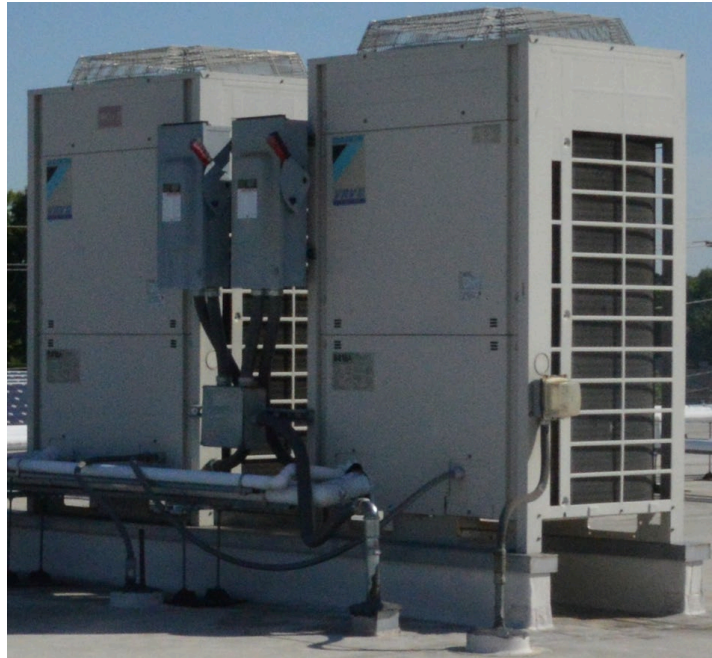
One of the 14-ton VRF heat recovery units mounted on the roof of the ASHRAE headquarters building.
